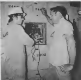
Employee Harry Koolman (r) observes student Etraín Kelly at work here in the NFAR switchroom.
